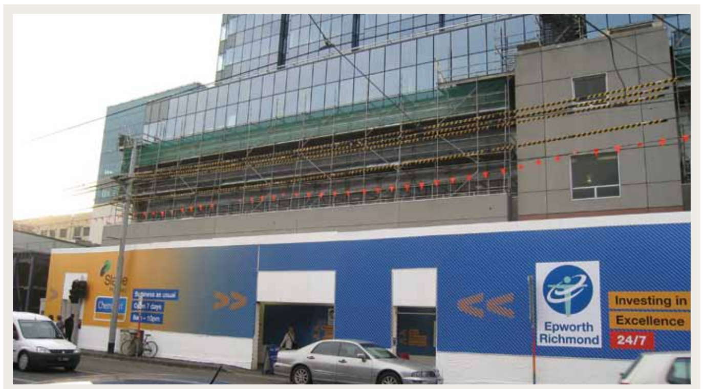
(Above left) Works to the Bridge Road Tower continue to progress. (Above) The external hoardings outside the Bridge Road main entrance are now visible
